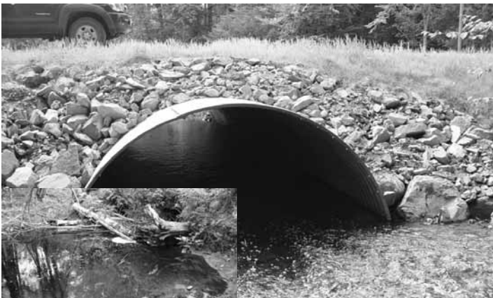
Rolfe Brook arch. Inset: clogged culverts at site in 2006.
